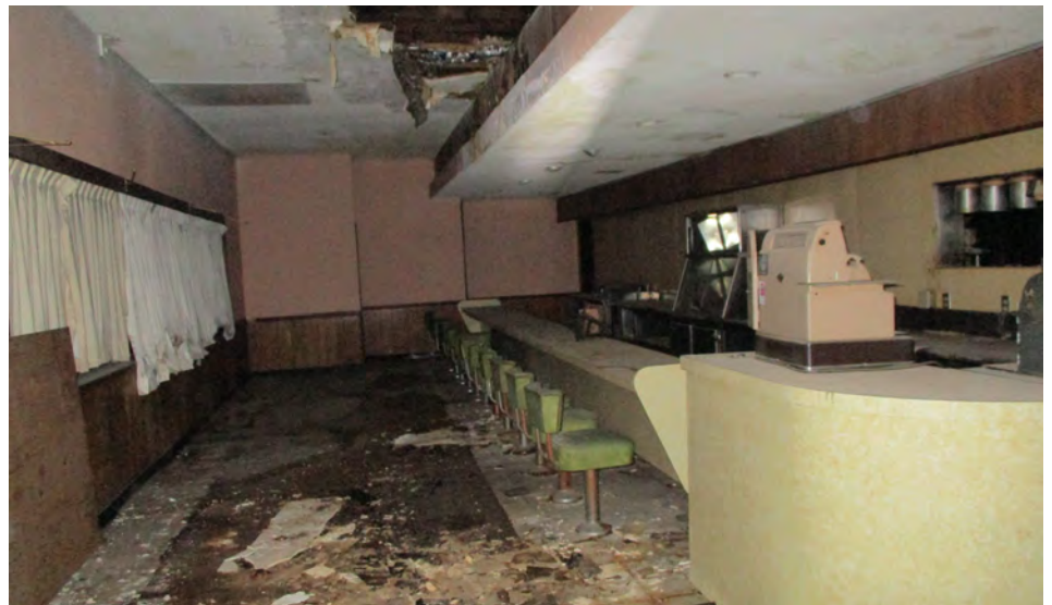
Café with collapsing ceiling, mold, wet floor
